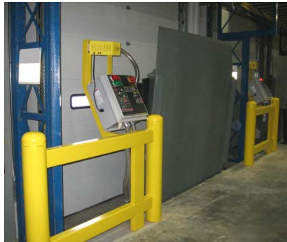
In the stored position, VSLs keep fork trucks away from the doors when not in use. Controls for the VSL, doors and other equipment can be mounted within guards that are built to prevent fork lifts from driving into the pit area.
