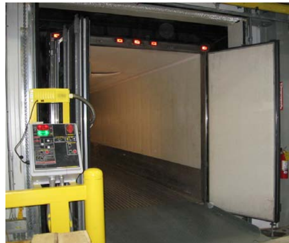
Drive-through docks with VSLs enable truck doors to open when inside the facility, while preventing many of the common injuries associated with forklift use on the dock floor.
